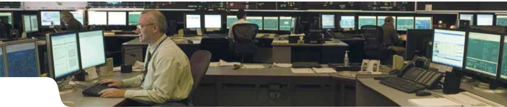
▲ IESO Control Room
